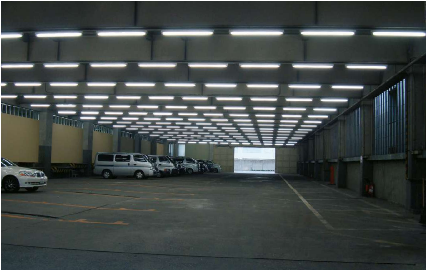
Industrial emergency luminaires
